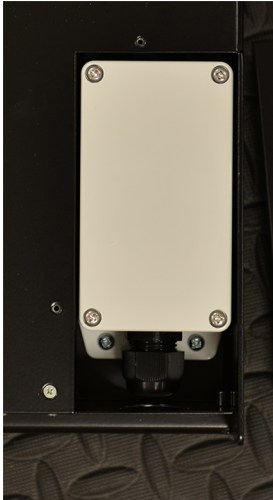
Figure 3 Exposed Power Box with rear panel removed.
